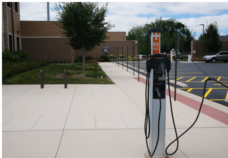
Electric Vehicle Charging Station at City Hall
